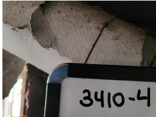
3410-4 Duct Wrap/Off-White (35% Chrysotile) Interior Air Handler (Appx 2 lin ft)
